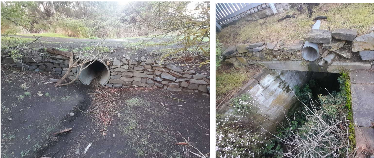
Figure 9. (L) Culvert under paddock access at Dysart House (R) Culvert under Main Street
