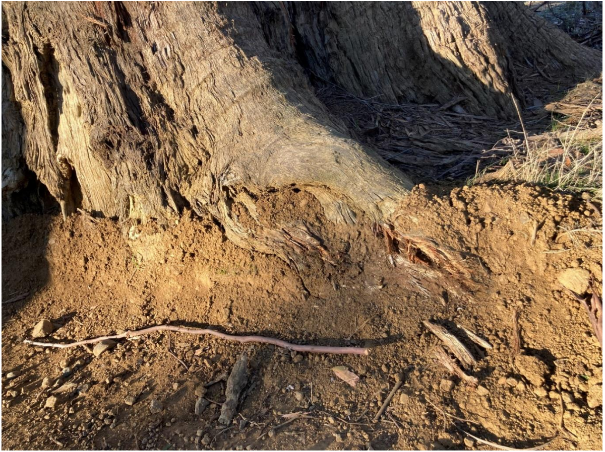
Figure 8 - T2 - Western side adjacent to Huntingdon Tier Road, showing apparent road-grading damage to the root buttress.
